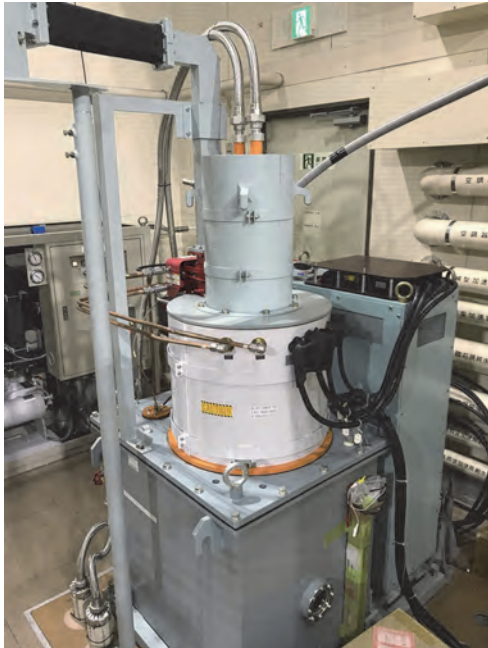
Fig. 3 New pulse transformer for the klystron modulator of the linac.
